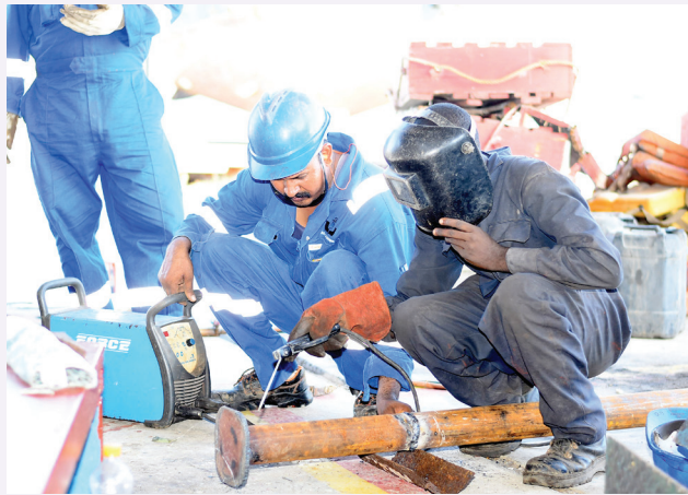
Marine welding Trainees in dual training 1 st industry block for 3 months in African marine and general engineering company.
